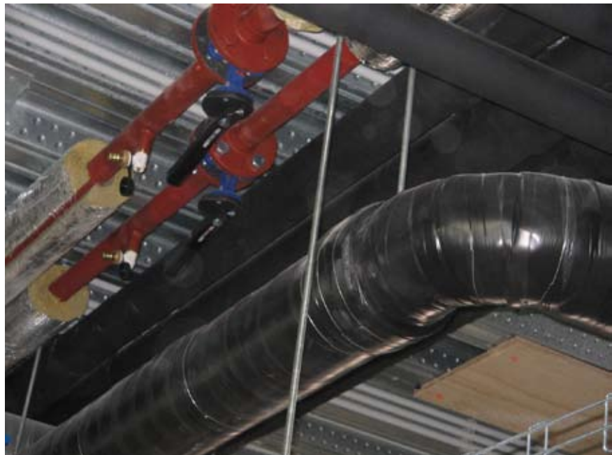
Merfolood on a pipe line
