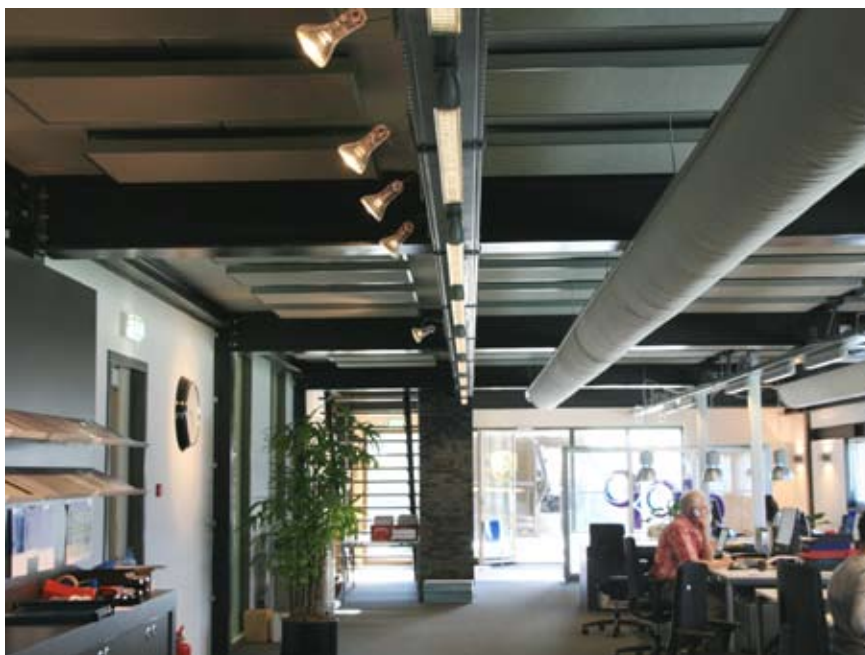
Soundstone baffles, kantoorpand DPP
